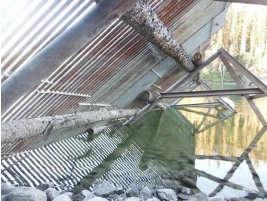
Figure 5. NB diversion weir in place (2013 photo). Note: Photo taken in late August at lower water levels than photo in Figure 4.
