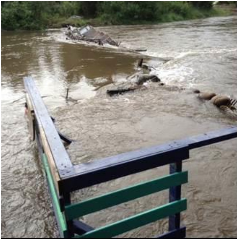
Figure 4. Collapse of fence structure, July 29.
