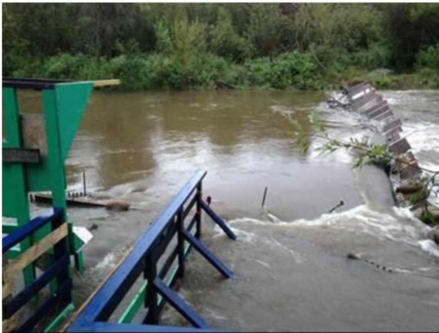
Figure 3. Flood conditions, July 28.
