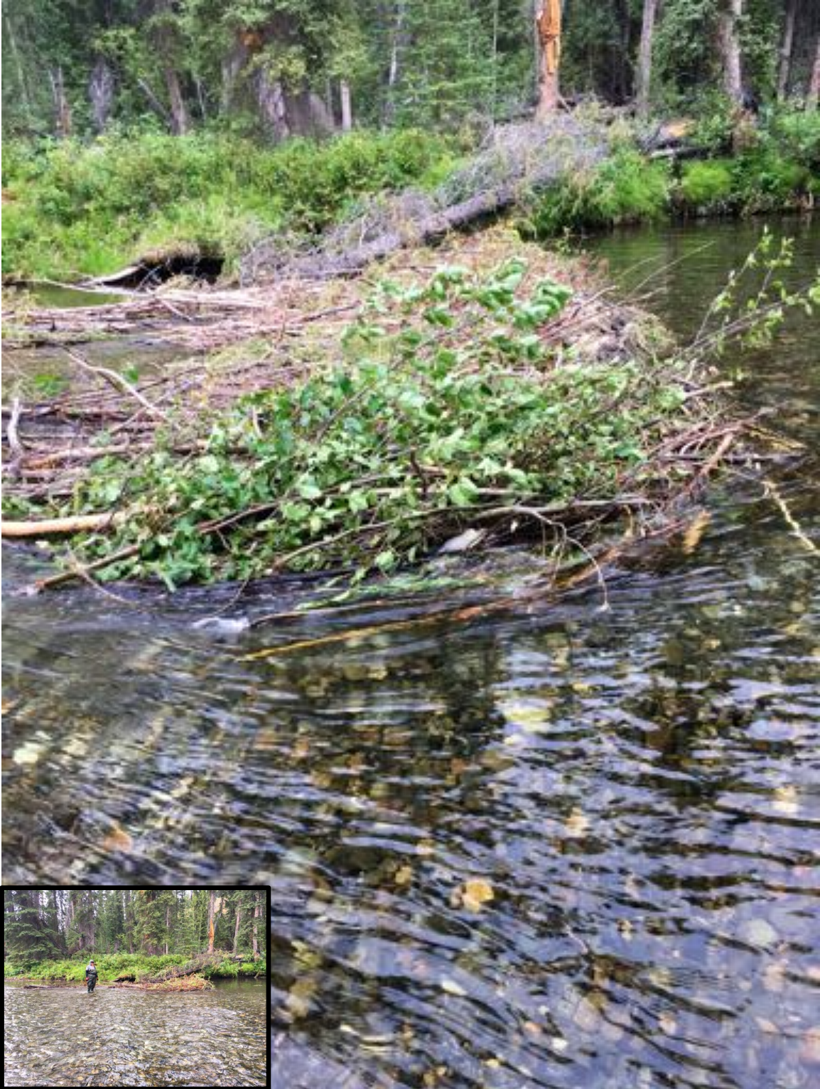
Figure 8 Before and after (insert) photos of the removal of a beaver dam situated in the primary spawning area of upper Michie Creek.
