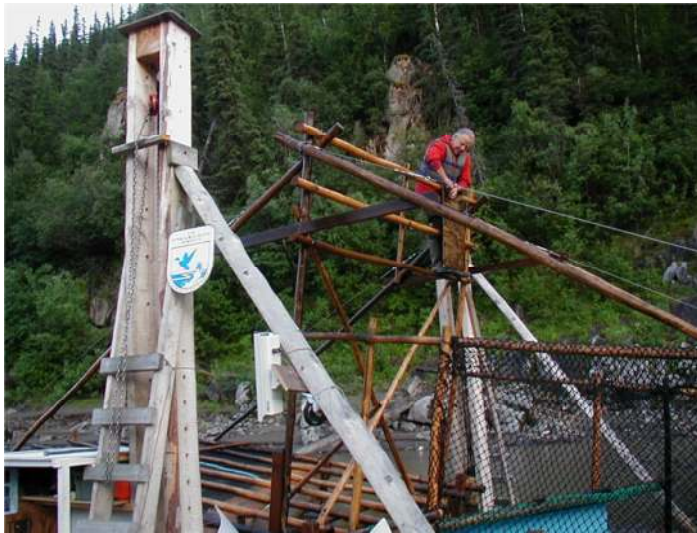
Changing paddle boards to keep wheel rotation slow for fish friendly operation.
