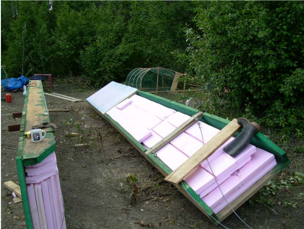
Photo 1. Detail of pontoon
