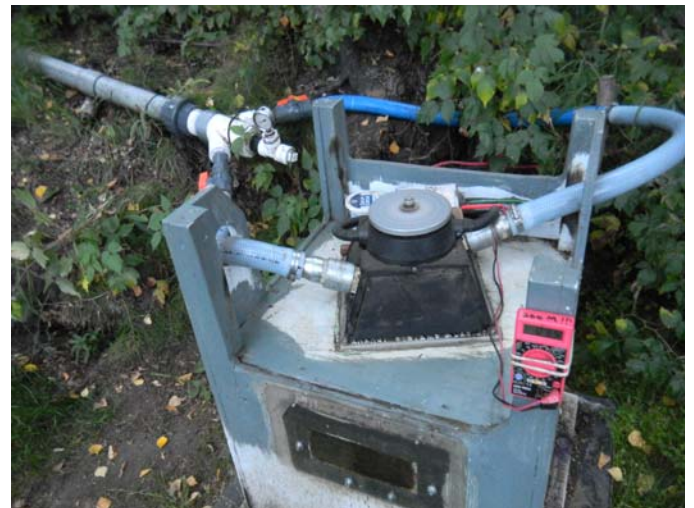
Rapids Research new water power system at main camp, 2011
